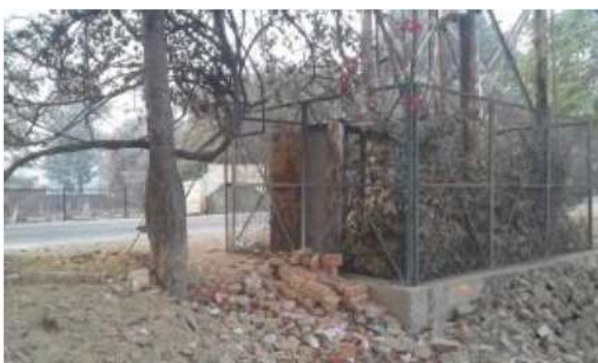
Transformer near the site towards 18M road
