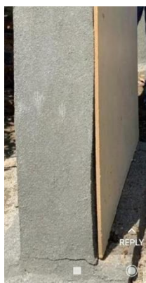
Fig.6.1 Failure of Double Brick Wall without Channel
