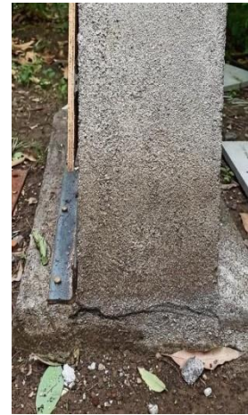
Fig.6.2 Failure of Double Brick Wall after attaching channel
