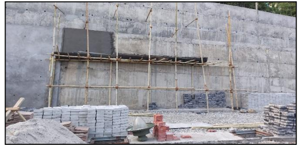
Figure 13: Using of GG Road tiles at roadways for looking better and controlling the slippery of prevention as per slope calculation beside the building structure
