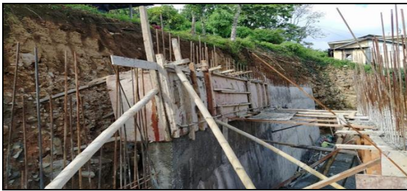
Figure 16: RCC Retaining wall construction but very bad lapping joint & finishing work is not well from outside to inside
