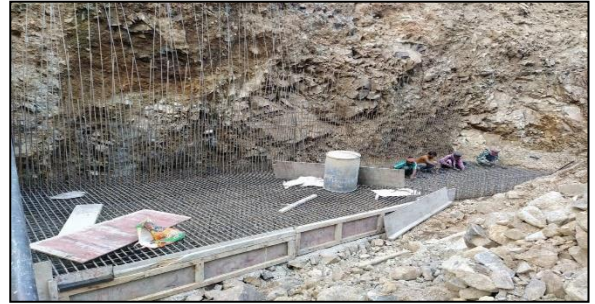
Figure 12: Working on RCC retaining wall basement structure toe with stem for protecting landslide at site areas
