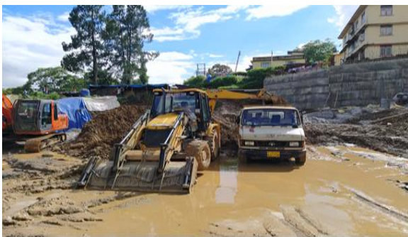
Figure 4: Site clearances after heavy rain & landslides using JCB & Tata and finishing the area plain for work
