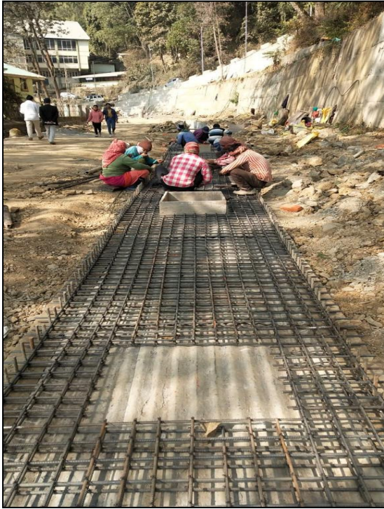
Figure 10: Working on RCC work for underground top Level slab casting of drainage line
