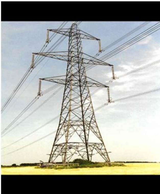
Figure. 1- Transmission line tower
