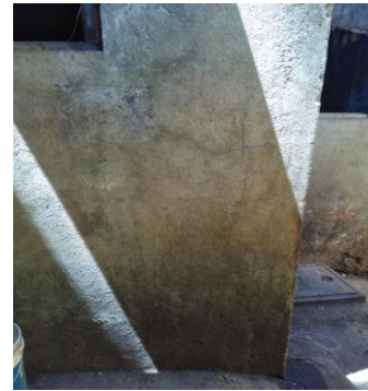
Fig. 1 crack width 1-1.5 mm is found.
