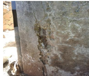
Fig. 2 Exposed reinforced found in column.
