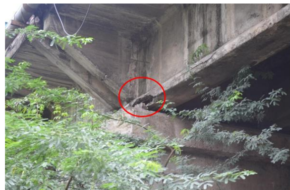
Image- (e): damage to the structure at bearing location
