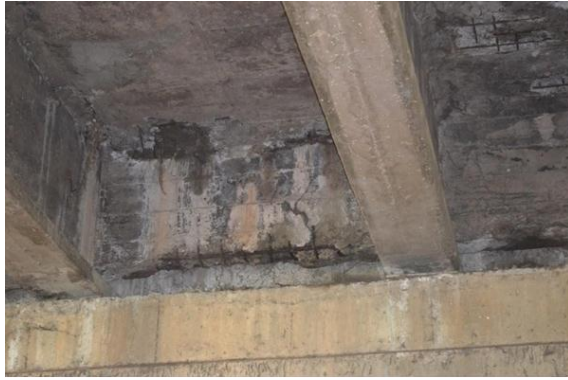
Image- (f): Damage in deck slab, steel is open in slab
