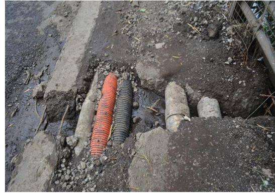
Image-(b): service lines in footpath are not covered
