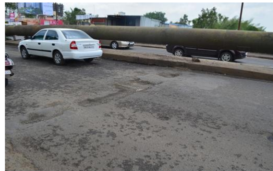
Image-(c): Expansion joint are to be damaged
