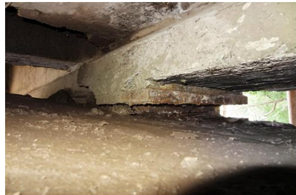
Image-(d): Damaged bearing
