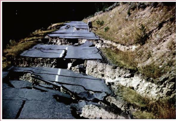
Figure 6: The 1959 Hegben Lake earthquake caused lateral spreading damage to roadway street in Yellowstone Park (photo courtesy of the USGS).
