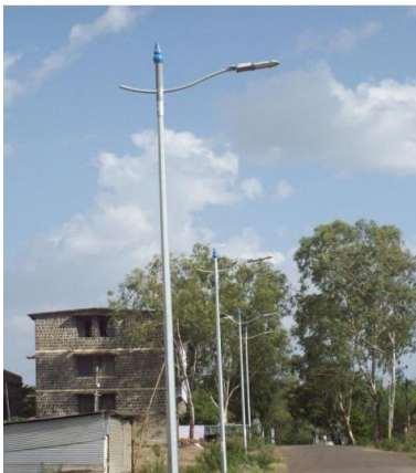
Fig.5. Street lighting near staff quarters of campus
