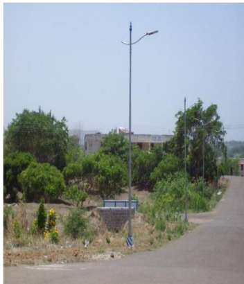
Fig.6. Street lighting along approach road of campus
