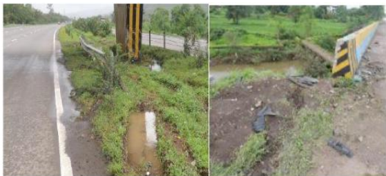
Unguarded bridge pier
