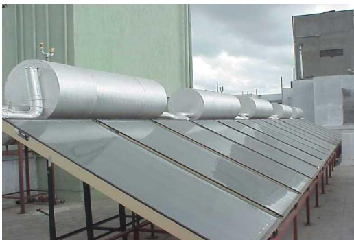
Figure 6: Water Heating by Solar System in City
