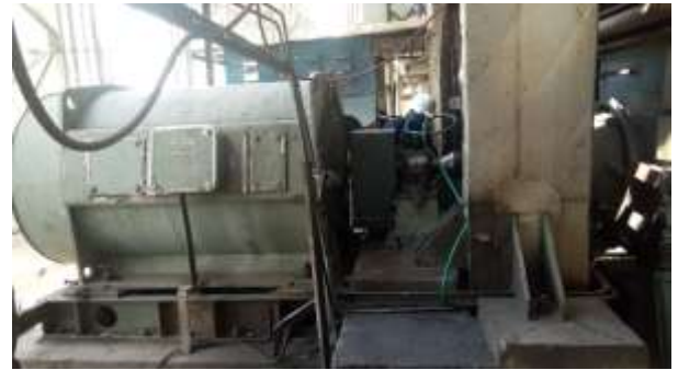
Figure 5.1.1(a) Side view of the SC Fan
