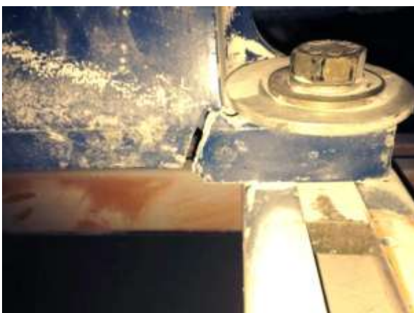
Fig .4.1.2 Crack in bench near foundation bolt.
