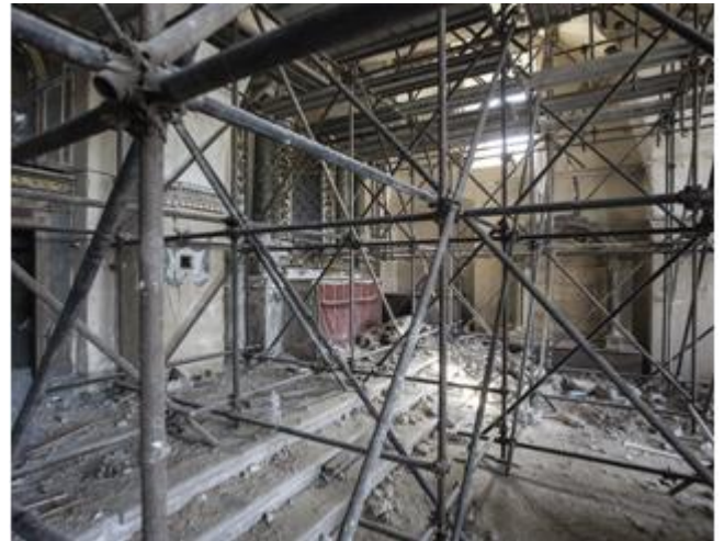
Church of Sant'Andrea in Campi di Norcia; the presence of rubble and securing made laser scanner survey operations difficult.
