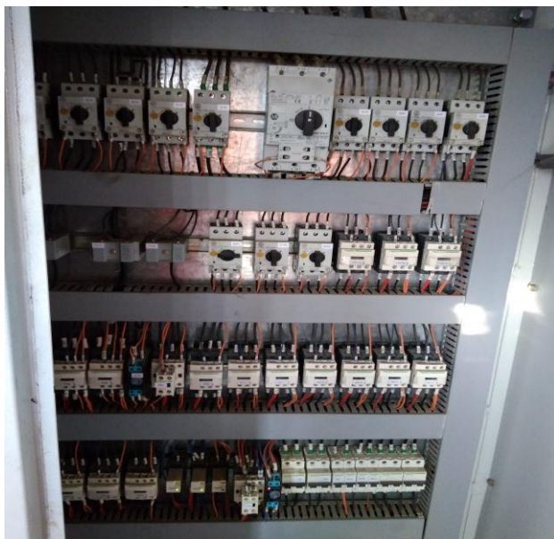
Figure4. SCADA Equipment control panel
