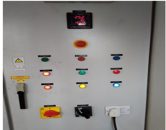
Figure5. SCADA Equipment control panel
