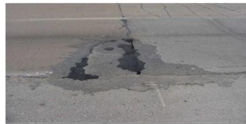
Figure 2. Shows developed cracks of deck surface
