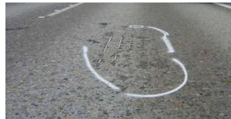
Figure 1. Shows surface Damage and repair of bridge
